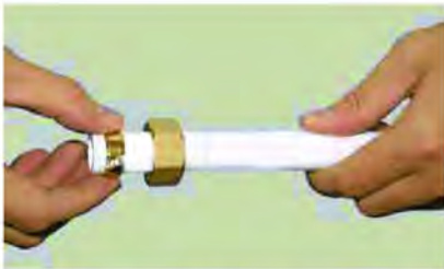
3. Choose the right size fitting according to the pipe, put the nut over the pipe, slide the compression ring over the pipe, make sure the mouth of the nut and the pipe faces the same direction.
